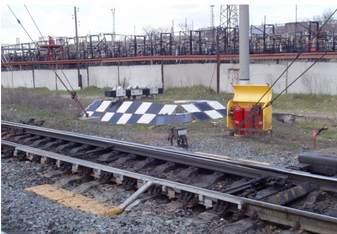
Gas-powered railroad switch heating system installed near Saratov, Russia.
