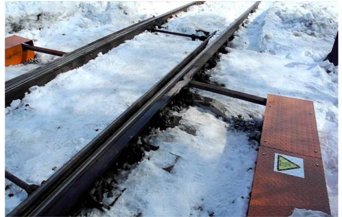
Gas-powered railroad switch heating system.
